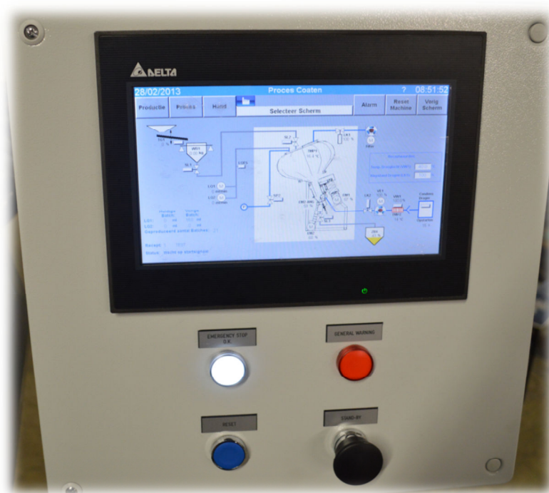
Complete process overview with 10" HMI
